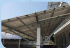
Carports (Welding type)
