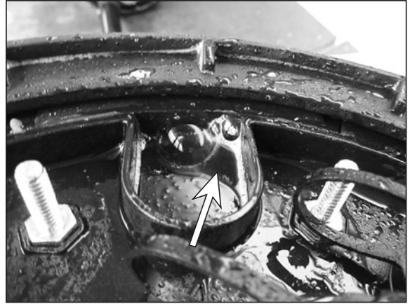
Leak occurring at the corner of the cable port
