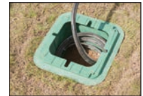
Slack Cable Storage in Small Base
