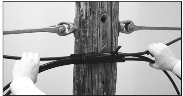
FIGURE 6: ABRASION PROTECTORS GROUPED WITH CABLE STRAPS AT POLE.
