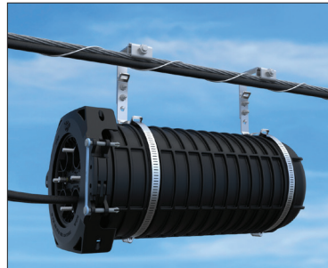
Completed Installation for Strand
