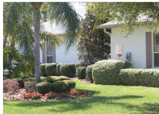
MPC Mounted to House
