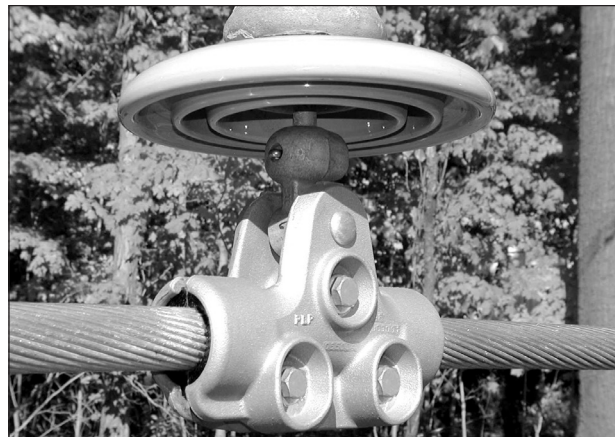
Completed application of the CUSHION-GRIP Suspension. The work hole located on the bottom of the clamp have a maximum working load of 500 lbs.
