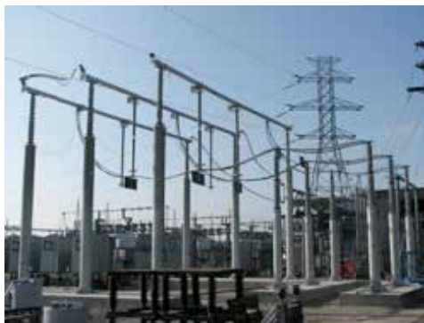
FULL SCALE SHORT CIRCUIT TESTING TO 63 kA/1sec POWERTECH LABORATORY, VANCOUVER, 2009.
