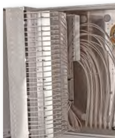
Cable/duct management view
