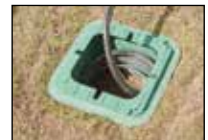
Slack Cable Storage in Small Base
