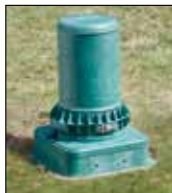
Installed 17" (453 mm) GLC with Grounding Spacer
