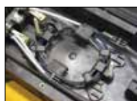
Installed Fiber Organiser for Ribbon
