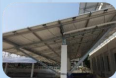
Carports (Welding type)
