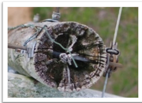
Pole rot with exposed through hardware
