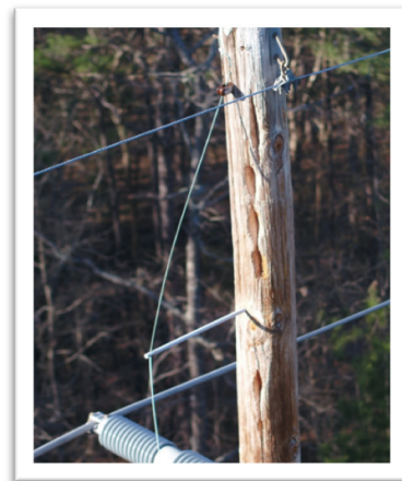
Repeated woodpecker damage
